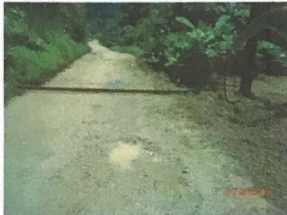
Stake Marks 25 Foot Boundary at Right, Road Cross Section is Flat (No Crown)
