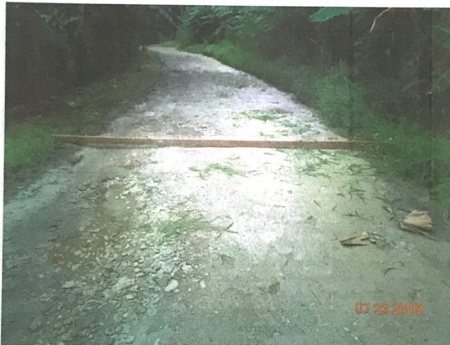
Erosion of Fines at Left side. Loose Gravel Remaining. Road Width Approximately 15 feet. Road Cross Section is Flat (no crown)
