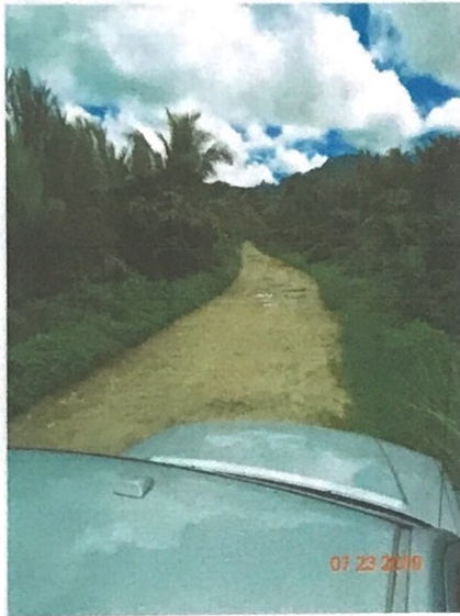
Depressions in Roadway
