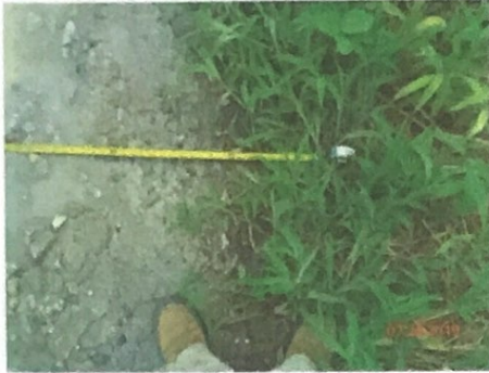
Roadway Down to 10 Feet Wide at Culvert
